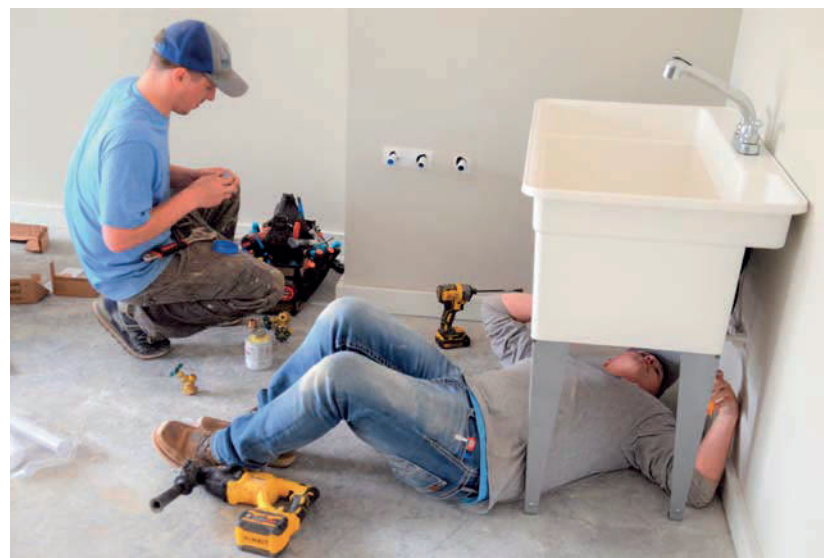
From left, Jack Fitzgerald and Ben Munson work at installing a sink at a new construction in Annandale.
